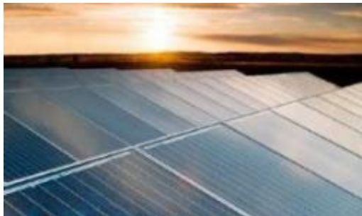
White Bluffs Solar Station (38 KW)
