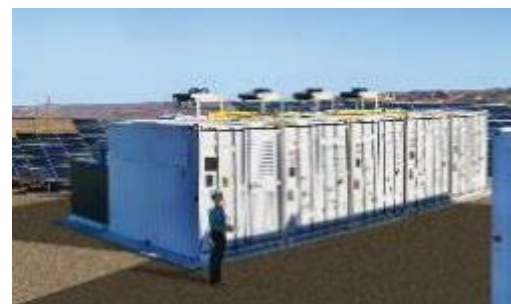
Horn Rapids Solar, Storage & Training Project (4 MW)
